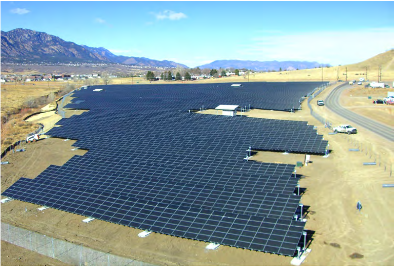
Solar photovoltaics at Fort Carson, CO
