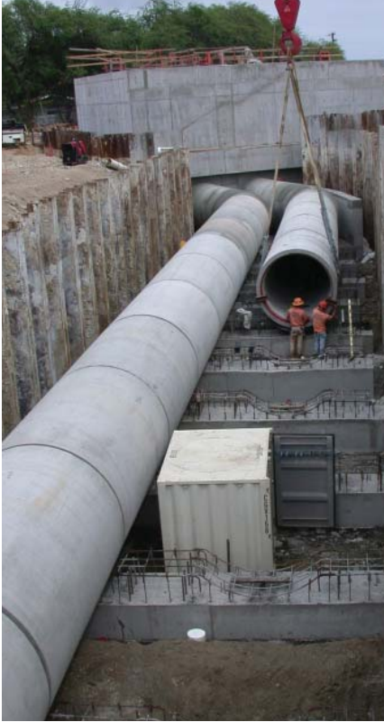
Approximately 17 feet below grade, and 9 feet below the Pacific Ocean, Parsons mechanical crews lay a twin-78-inch reinforced concrete pressure pipeline on top of a jet-grouted trench bottom.
