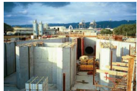
Looking at an influent 96-inch pipeline to the Screening Facility, Parsons crews have staged the falsework for cast-in-place walkways above the future wastewater flow.
