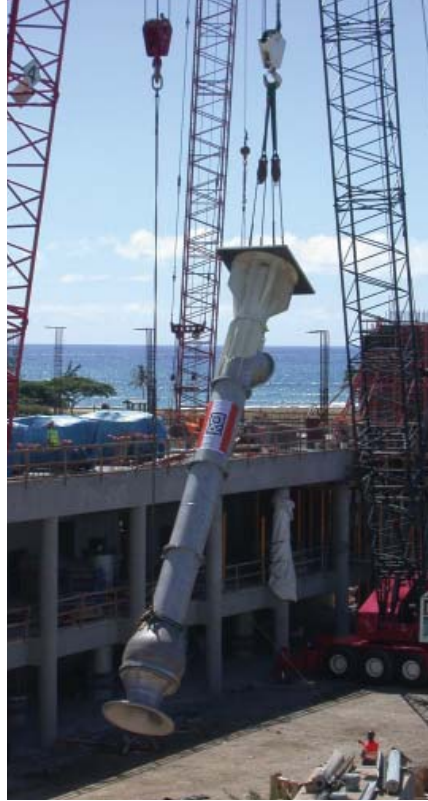
This 70,000 lb. vertical turbine pump shaft required two cranes to lift it off the ground. This first pump of four was successfully hoisted into its final location by Parsons crews.
