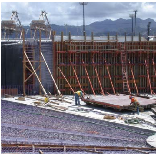
Parsons carpenters prepare an interior formwork panel for hoisting. This was the first of 72 wall pours for the two-each 140-foot diameter cast-in-place primary clarifiers.
