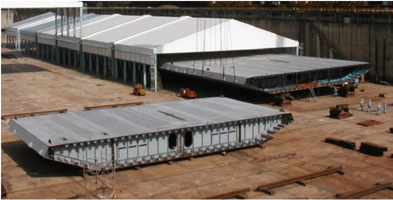
Superstructure box girder trial assembly progresses in the dry-dock prior to shipment to the Carquinez Bridge Site. A total of 24 box girder units will be suspended from the new main cables and welded together forming a 3,464 ft. continuous stiffening girder weighing upwards of 14,000 tons.
