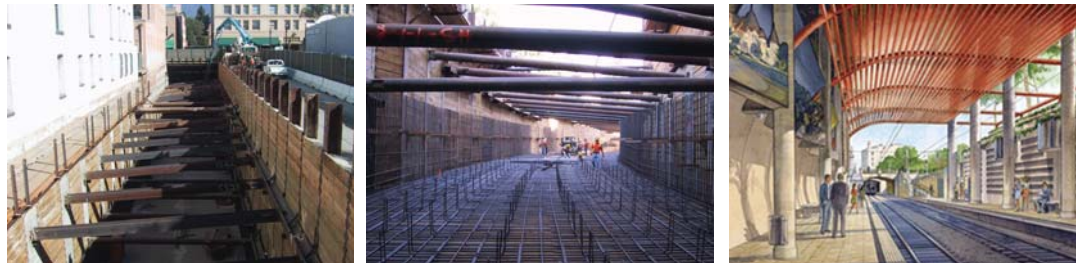
Left and middle: Construction at Colorado Boulevard Right: Rendering of Memorial Park station
