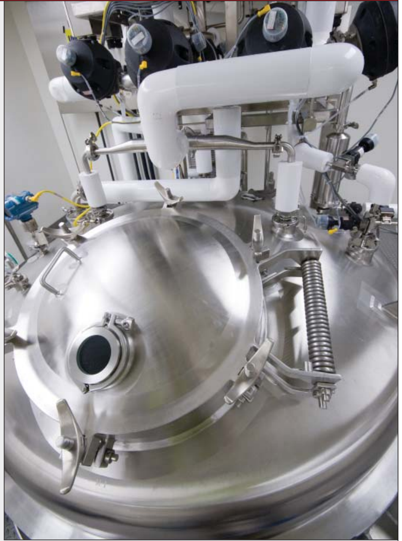
Top of a product-holding tank in LBXS1 purification suite
