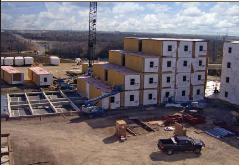
METC dormitories use modular construction with sections containing two rooms and a corresponding section of the central hallway—manufactured offsite, transported to Fort Sam Houston, stacked one on the other, and then bolted together onsite (photos courtesy of USACE).
