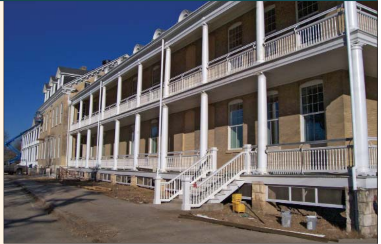
This 1908 hospital on Fort Sam Houston is being renovated to create administrative space (photo courtesy of USACE).
