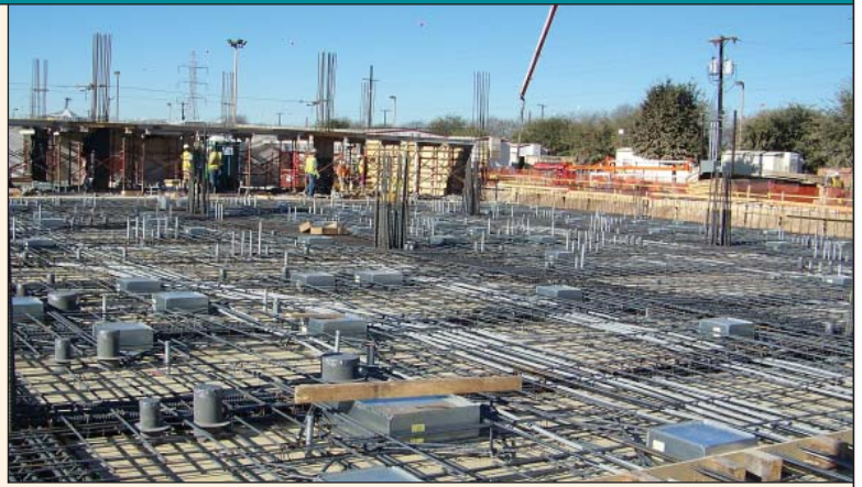
An expansive grid of rebar will support the 150,000-ft 2 Joint Center of Excellence for Battlefield Health and Trauma (photo courtesy of USACE).
