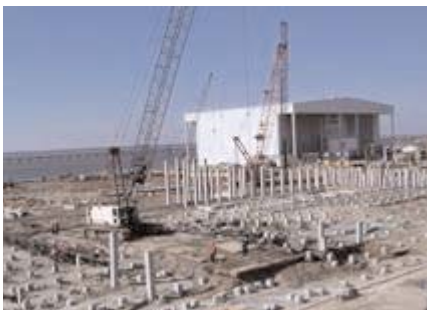
Ingalls' new ship erection area with existing blast and paint facility in the background.
