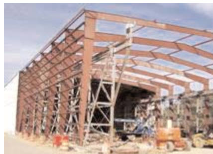
Expanded composite cutting facility at Gulfport.
