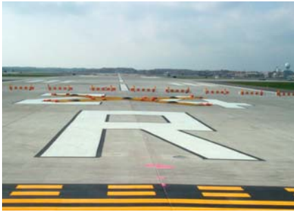
Runway ready for preflight checkout on November 11, 2002, one month ahead of opening day
