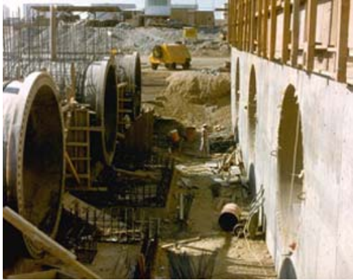
Seawater is distributed to Yanbu's industries by 27 kilometers of underground piping. Some of the pipe, like that pictured here, is nearly 4 meters in diameter.
